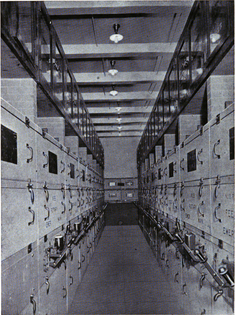
FIG. 144.—High-Tension Compartments, "K" Switch Side; Sixteenth Street Substation.
